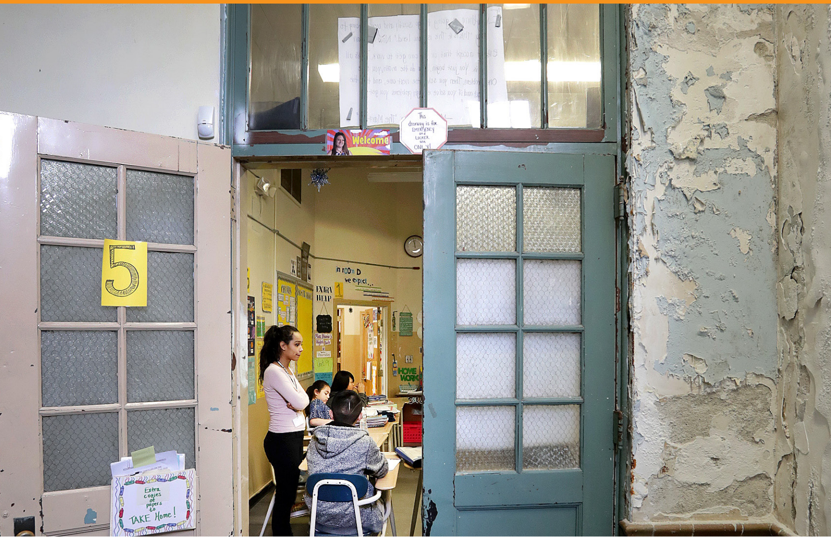
A deteriorating wall outside a classroom at the Pickering Middle School in Lynn, MA is pictured on Feb. 14, 2017. Photo by John Blanding/The Boston Globe via Getty Images
