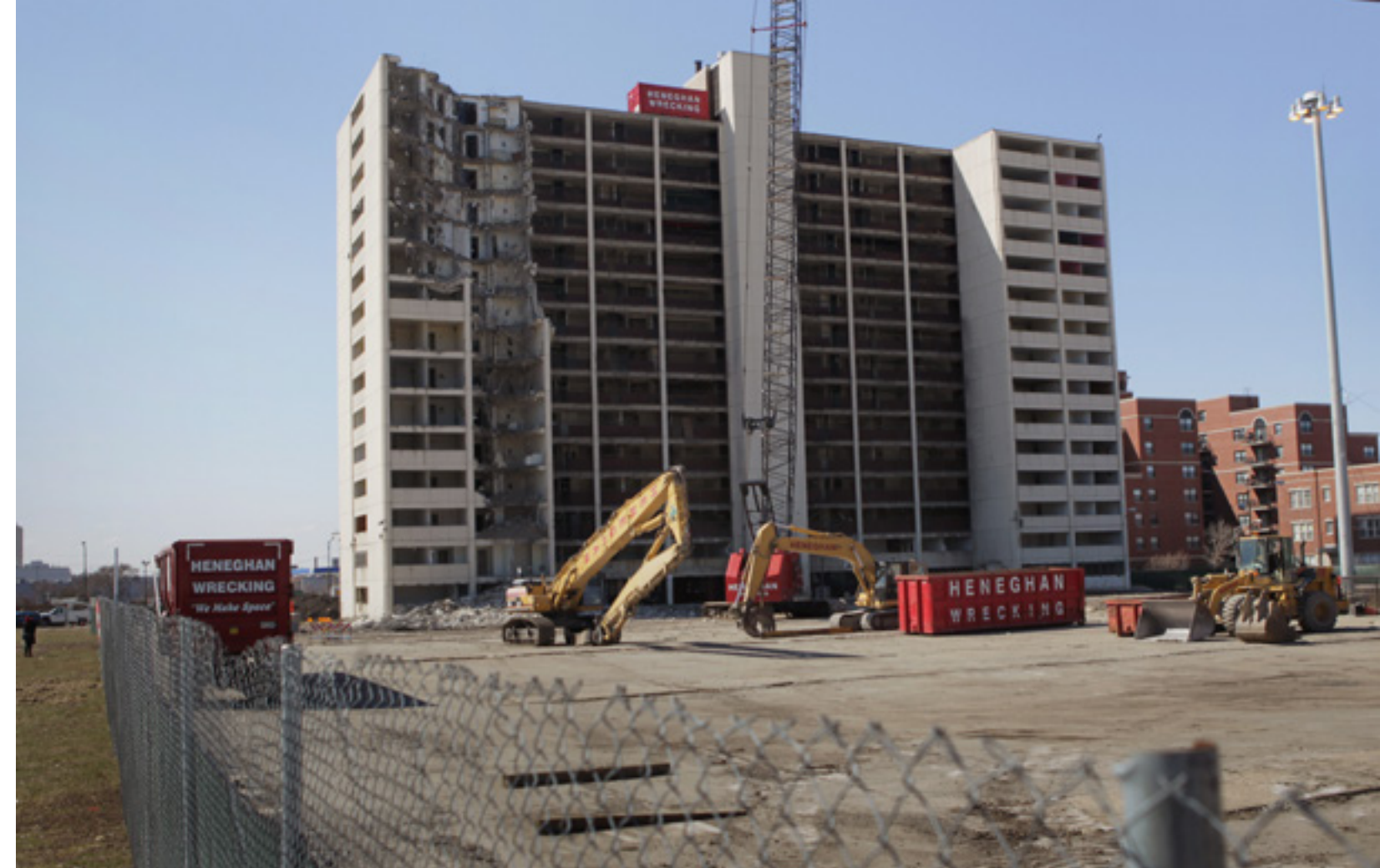
A wrecking crew begins the demolition of the last remaining high-rise building from the infamous Cabrini-Green housing project March 30, 2011 in Chicago, Illinois. Cabrini was knocked down in part because of the Gautreaux lawsuit. Photo by Scott Olson/Getty Images
